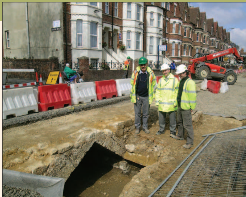
Fig. 16 A mitred arch belonging to the Norman Grandpont Causeway exposed in Abingdon Road in 2004.
