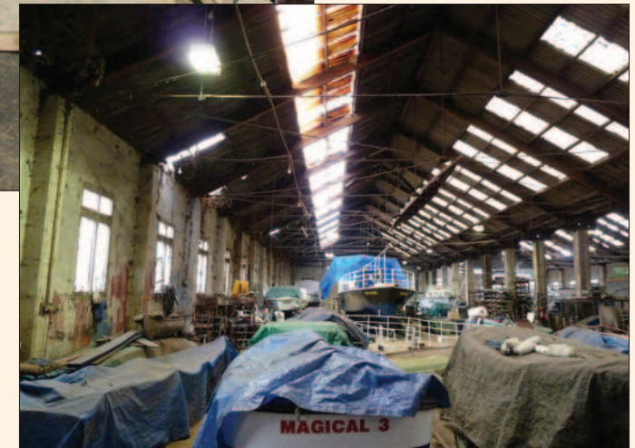
Fig. 32 Photograph of the Salters Steamers Boatyard at Donnington Bridge. Built in the 1930s and still in use as a boatyard.
