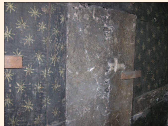
Fig. 30 Painted panelling and a door from a previously unknown 17th or early 18th century student study exposed at Brasenose College during building work in 2010.
