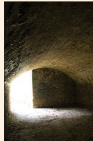
Fig. 28 A vaulted cellar and entrance chamber discovered in 2009 during building works at The Queen's College. Dated to the 17th century but perhaps containing fabric of earlier origin.
